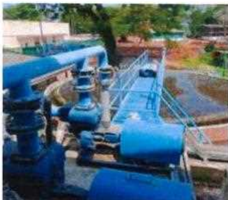
500 KLD STP at Kozhikode medical College
